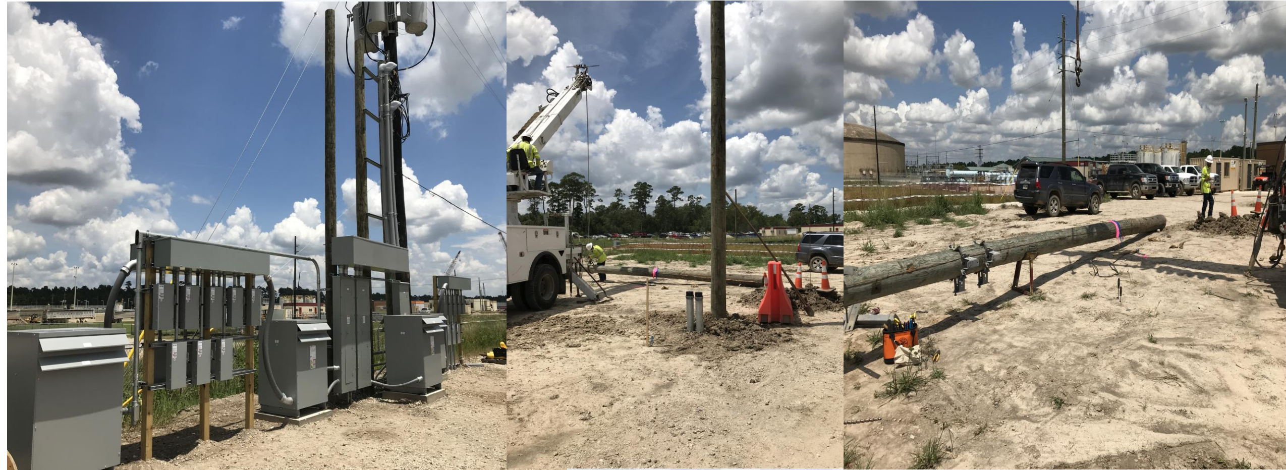
Trailer City 2 Complete 1200 Amps
