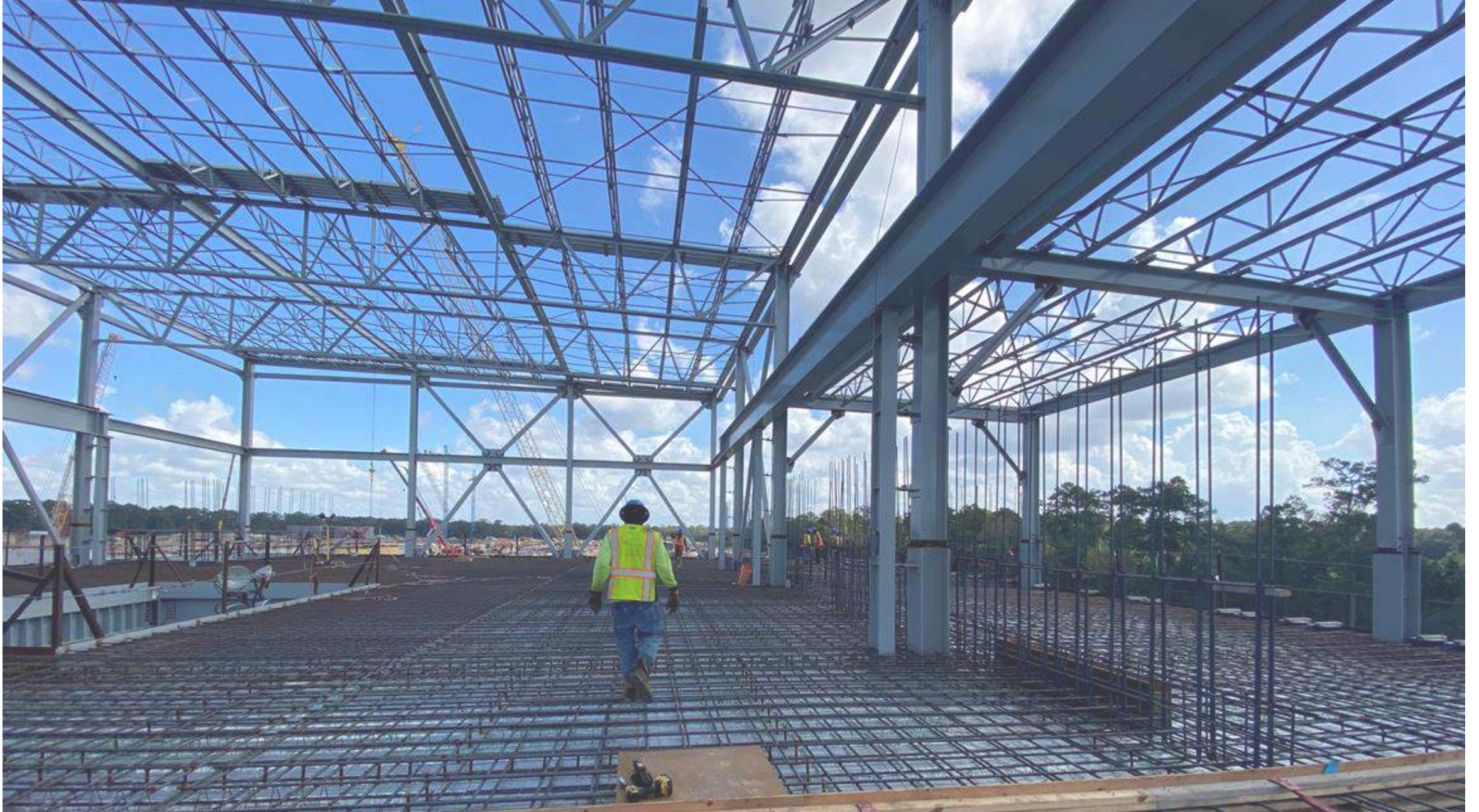
3rd Floor at Dewatering Building 520
