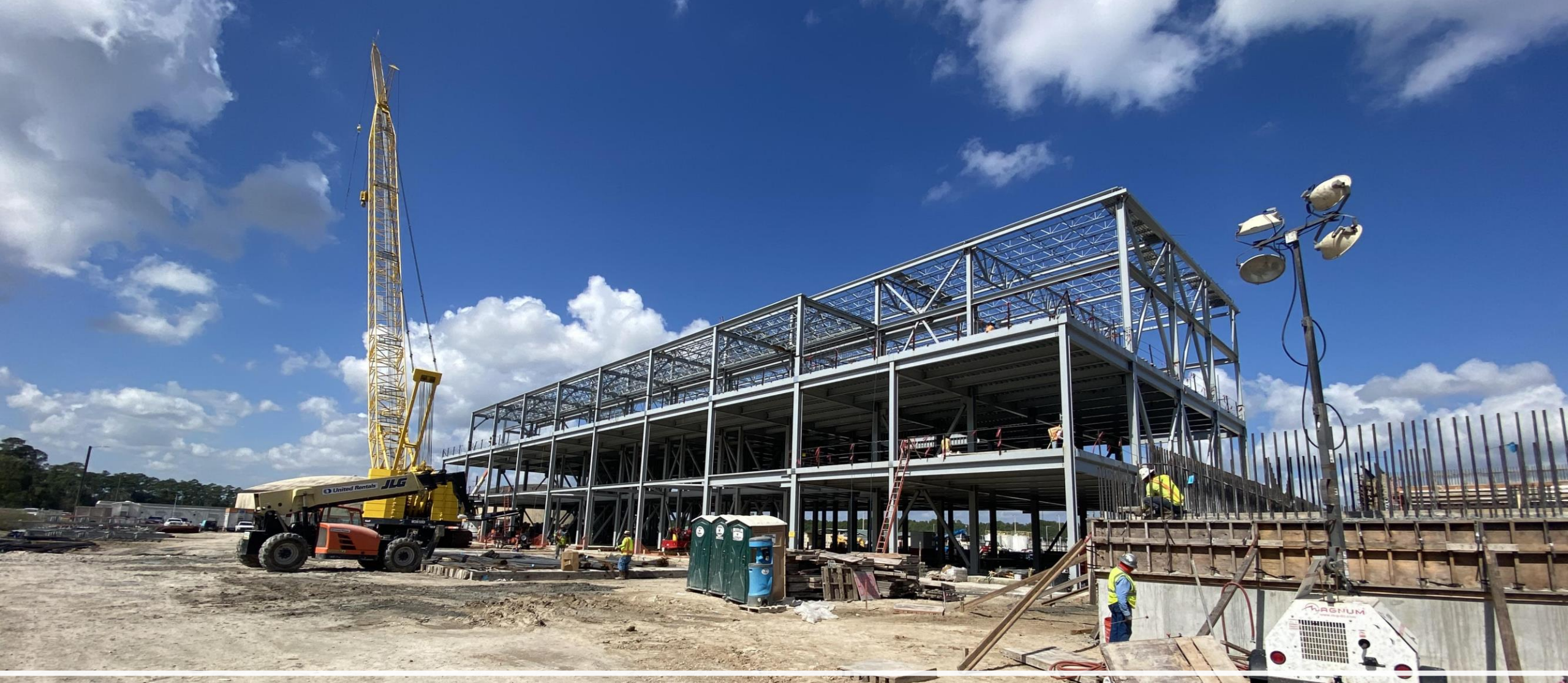
Rebar Installation at 3 rd Floor, grating installation at 2nd floor, and structural steel welding at the Dewatering Building 520
