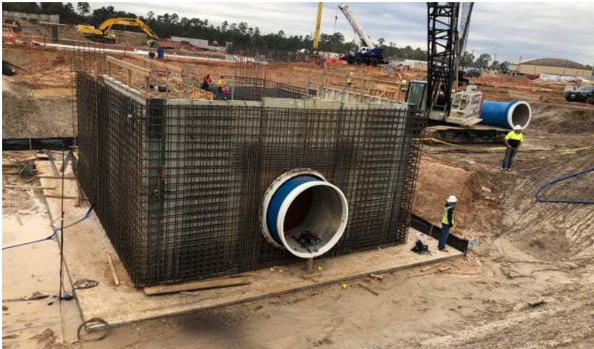
Facility 222 78" RW pipe penetration
