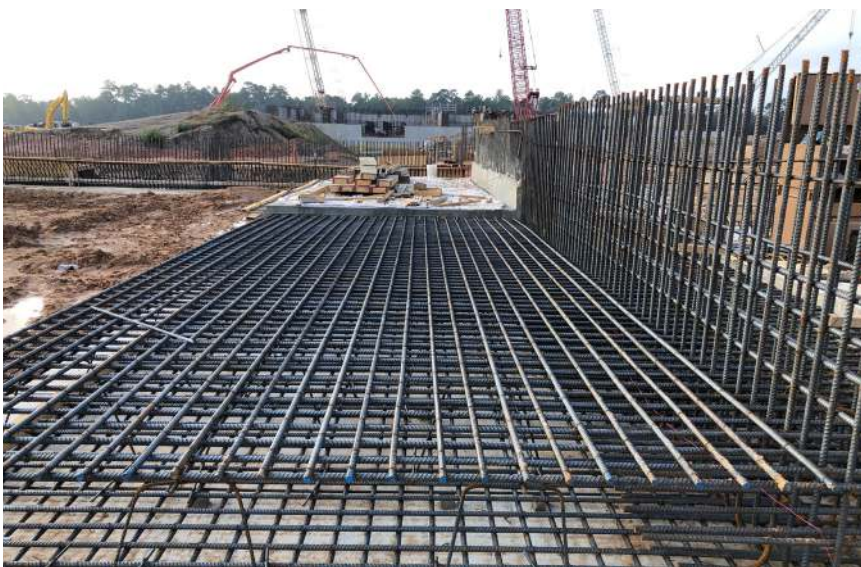
Facility 611 sedimentation basin
