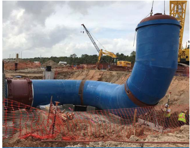
Facility 242 96 inch CW Pipe
