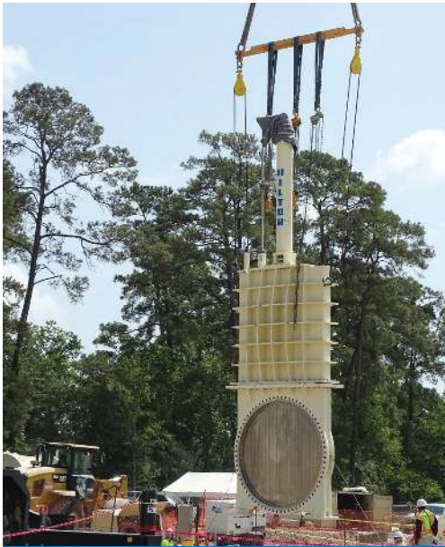
108" Knife Gate Valve in Corridor 1
