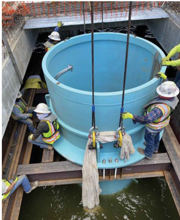
First Pump Can at IPS
