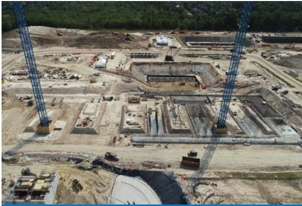
Central Plant – Phase 2
