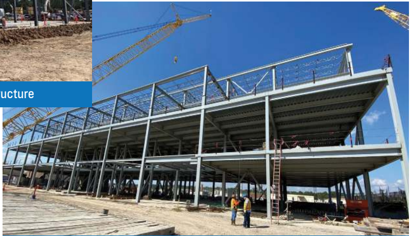
Erection of Structural Steel 3rd Floor Roof Framing at the Dewatering Building 520
