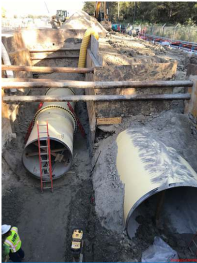
84" and 120" FW in Corridor 5
