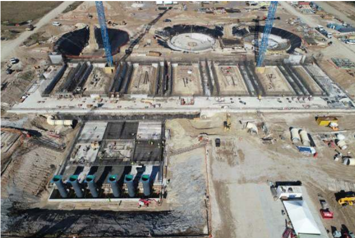
CENTRAL PLANT – 2nd Phase - Overall
