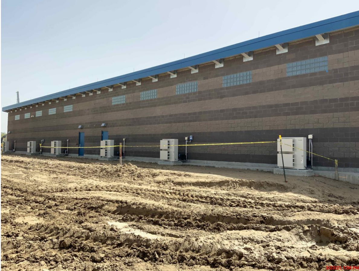
Ready to be energized with permanent power from Facility 102 ~
