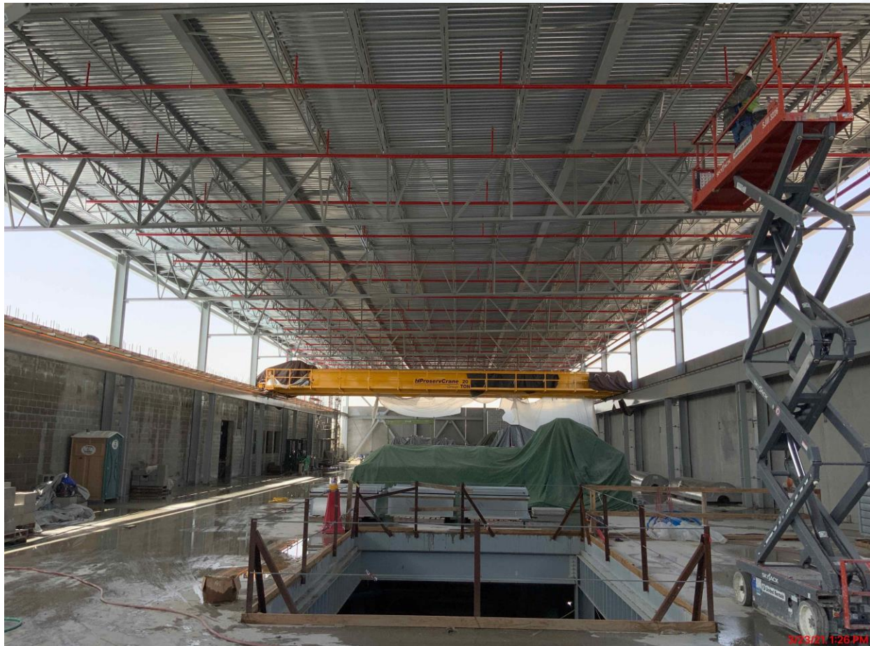
Continued installing fire protection piping on the 2nd & 3rd floor at Fac 520
