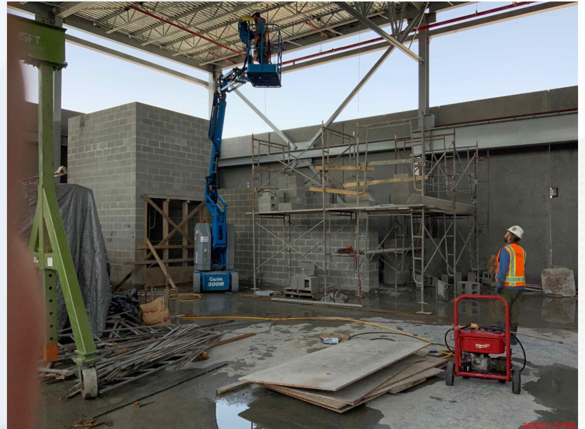
Commenced installation of CMU near the stairs at the 2nd and 3rd floors
