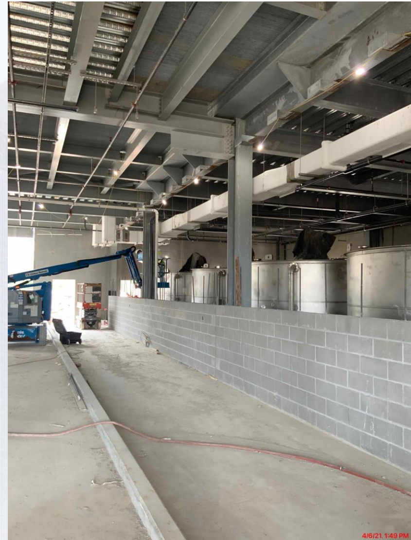
Continued installation of HVAC at the 1st, 2nd & 3rd floor at Fac 520
