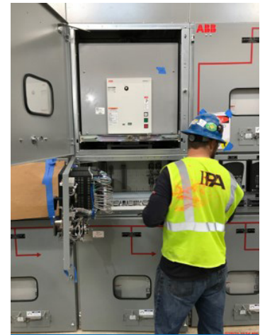
Function Test and Breaker Operation Facility 111 Main Switch Gear Building
