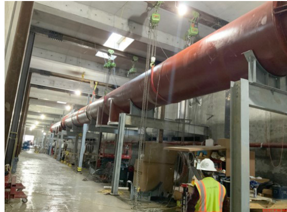
60-inch BWS Install Facility 281 Filter Module 1
