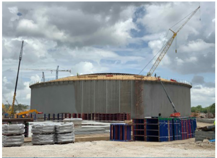
Shotcrete Facility 362 GST
