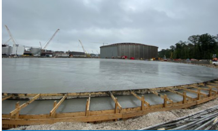
Ground Storage Tank 361
