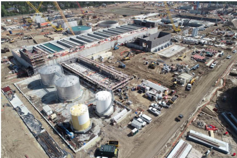
Central Plant - 1st Phase Overall
