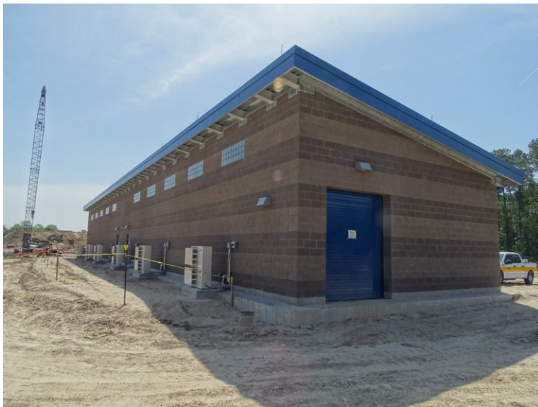
Main Switchgear Building 111
