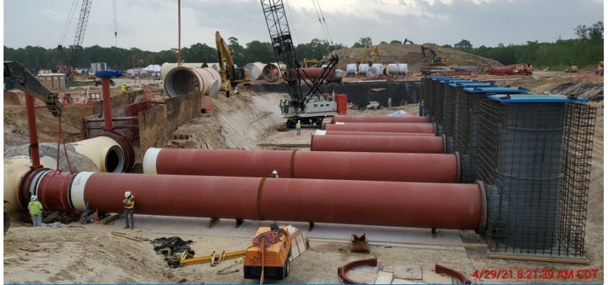
High Service Pump Station 402
