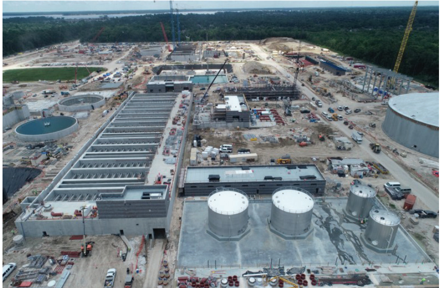
Central Plant- Phase 1
