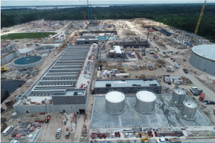
Central Plant - 1st Phase Overall
