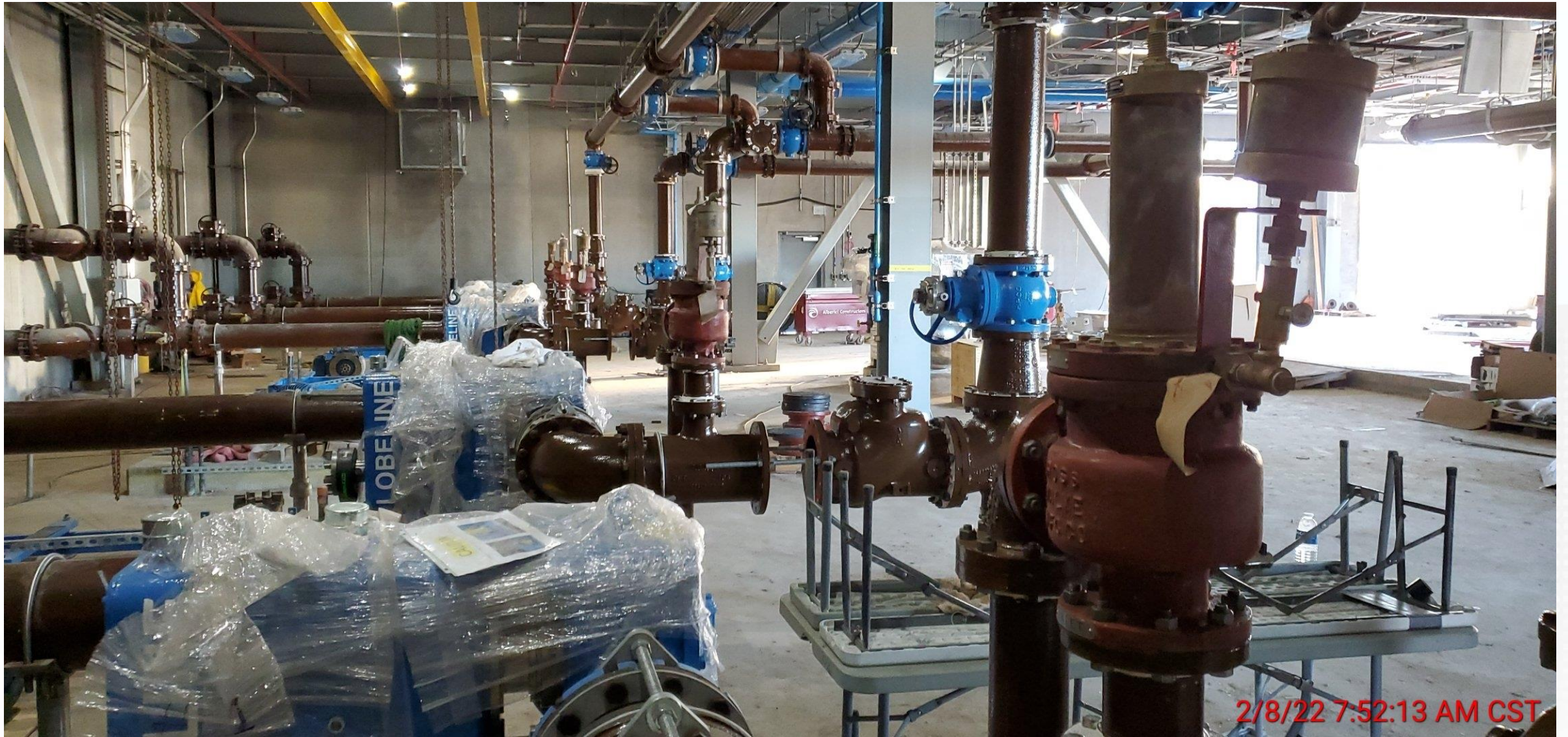
Continued installing plumbing, process pipe, and electrical conduit on levels 1, 2, and 3 at Fac 520.
