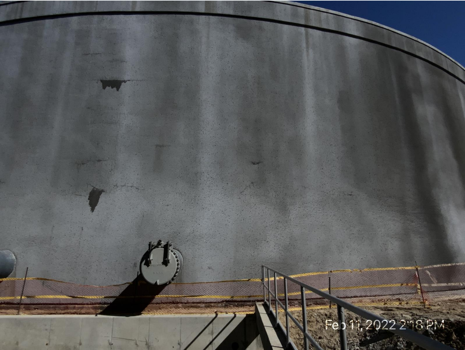
Passed watertightness test GST 362.
