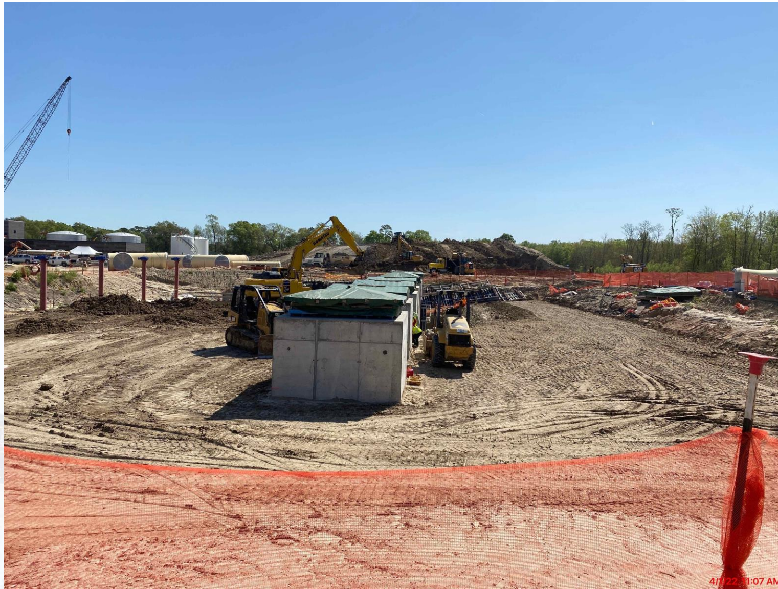
Continued backfilling and continued top of pump can encasement correction at Fac 402
