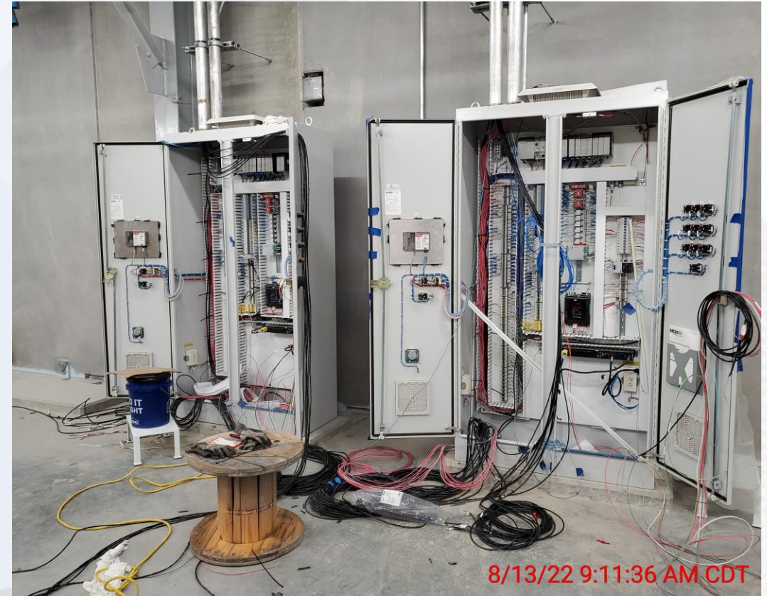
Wire Terminations in centrifuge electrical room
