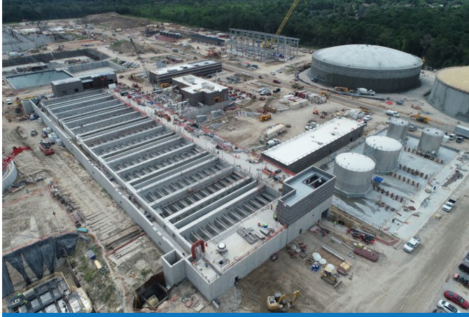
Central Plant - Phase 1
