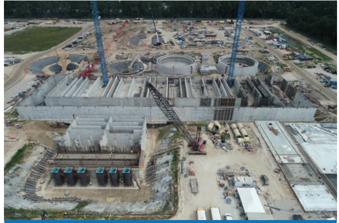
Central Plant - Phase 2
