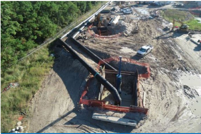
Corridor 1 – 42-inch HDPE Bypass Piping
