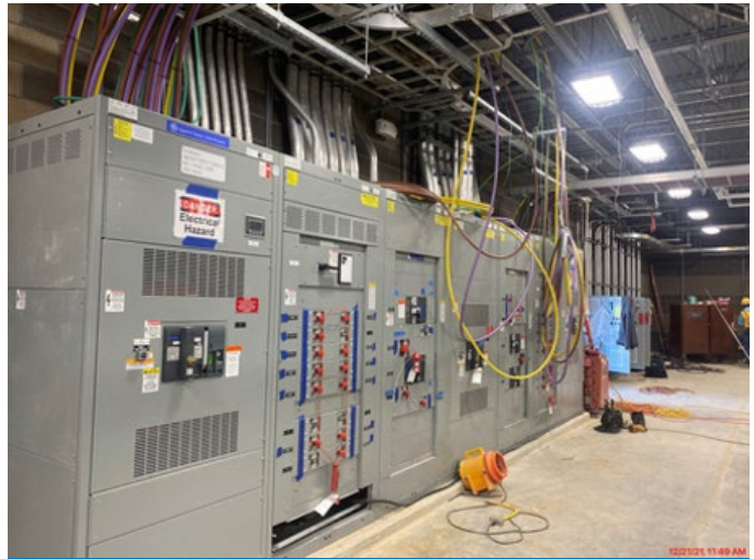
Energized Electrical Equipment Facility 291 TPS
