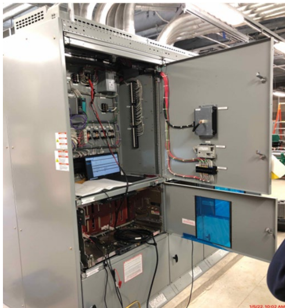
Third Party Testing Facility 401
