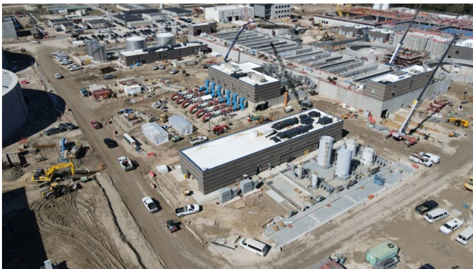
Central Plant – Phase 1
