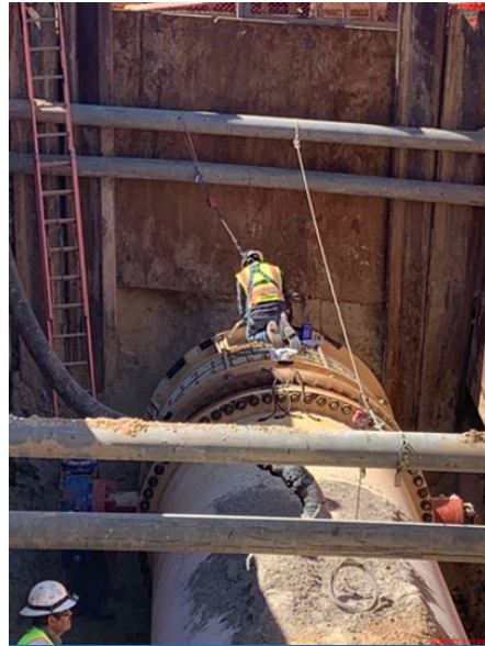
Air-gap Monitoring System: 96-inch FW
