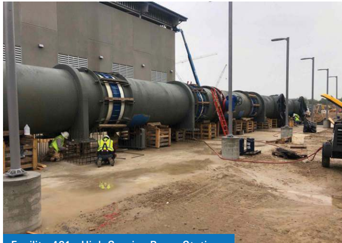
Facility 401 - High Service Pump Station
