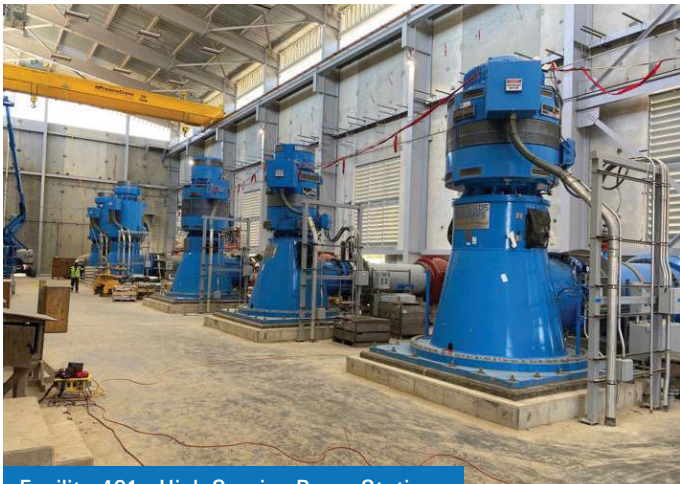
Facility 401 - High Service Pump Station
