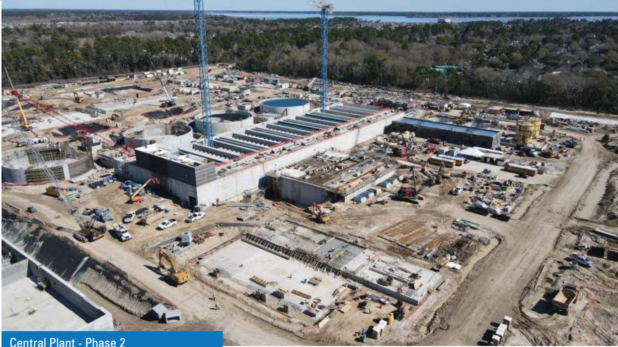
Central Plant - Phase 2
