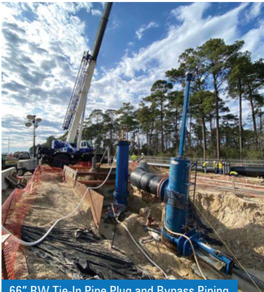
66" RW Tie-In Pipe Plug and Bypass Piping
