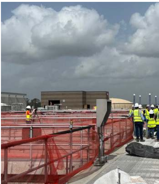
Facility 281 Filter Module - Equipment Training
