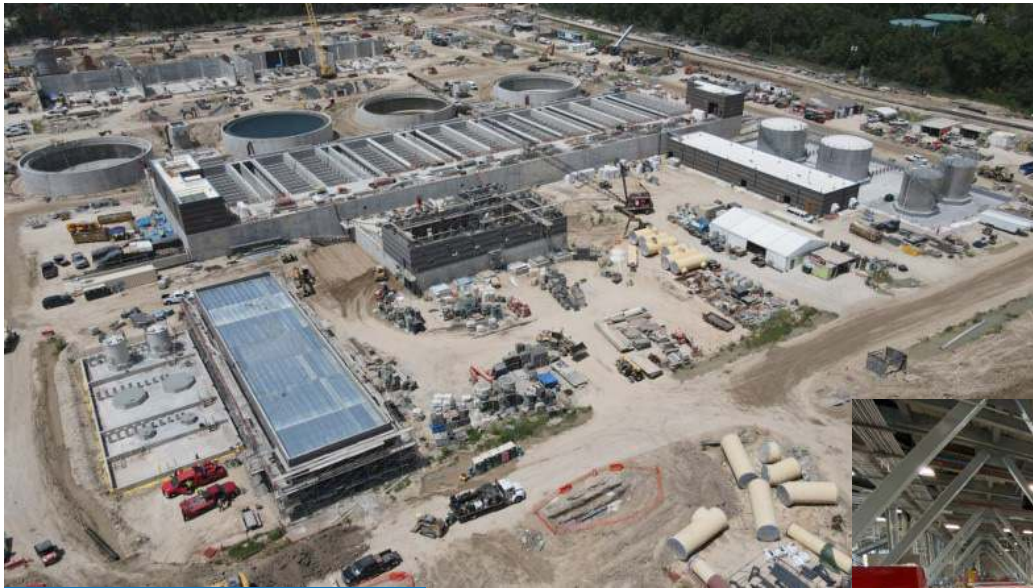
Central Plant - Phase 2
